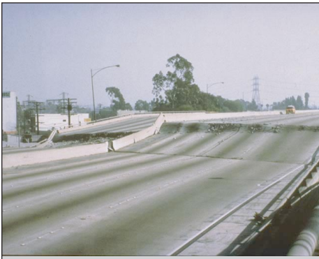
This section of the Santa Monica Freeway was severely damaged when the Los Angeles region was struck by the 1994 Northridge earthquake, the costliest quake in U.S. history. However, freeways of similar construction even closer to the source of the quake went unscathed. The Santa Monica Freeway was damaged because the ground beneath it amplified the shaking, causing the freeway to fail. (U.S. Geological Survey photograph by Mehmet Çelebi.)
